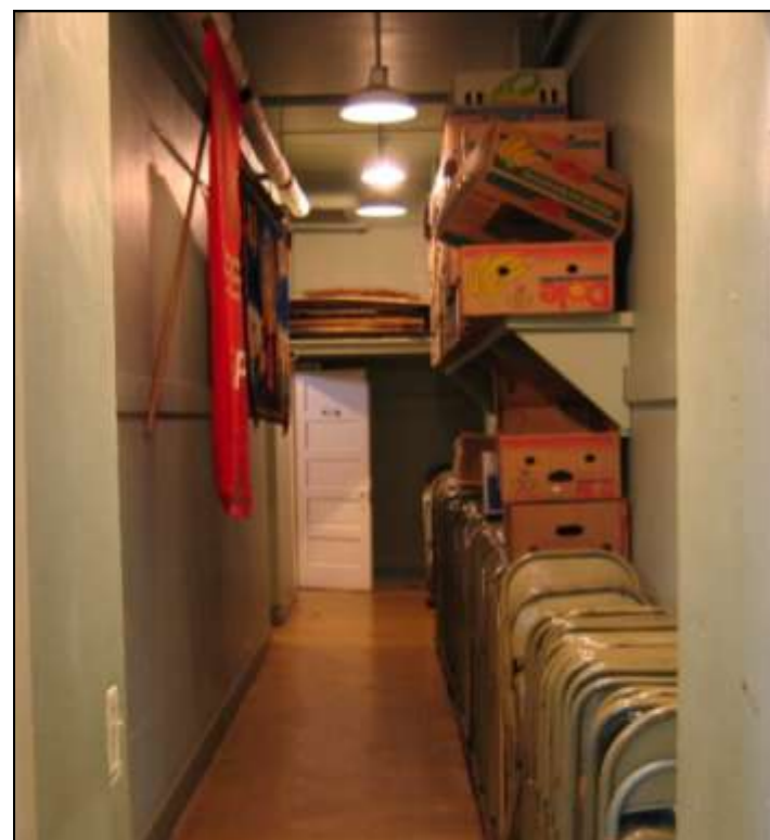
The tight entrance to the hallway will be expanded to accommodate the handicapped.
